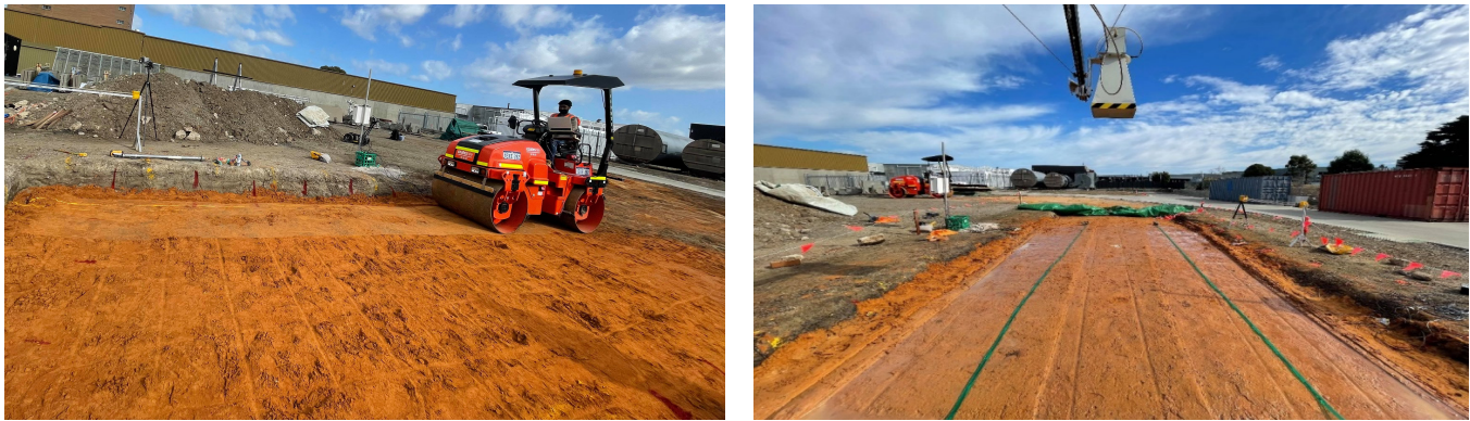
Fig. 3. Photographs showing (Left) compacting of the soil using a roller and (Right) watering of the surface using sprinklers.
