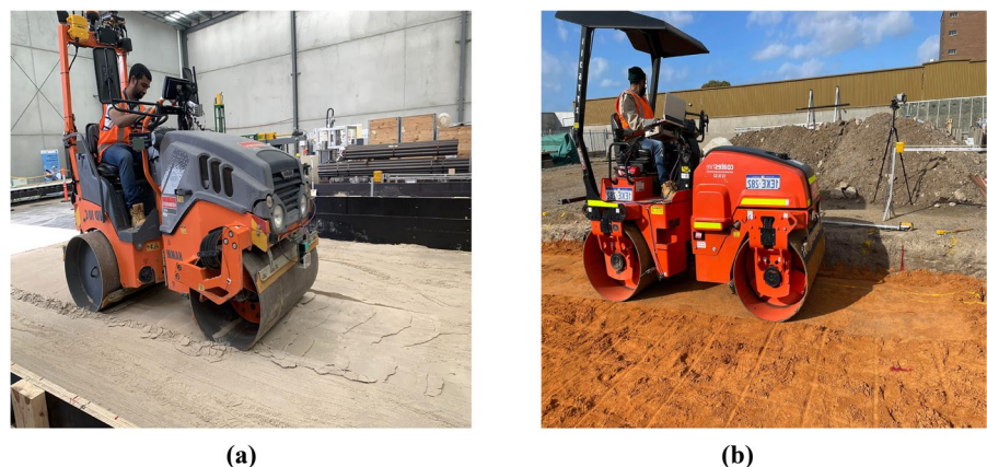
Fig. 3 Photographs showing the roller used to compact the soil at (a) the soil box and (b) the test-bed
